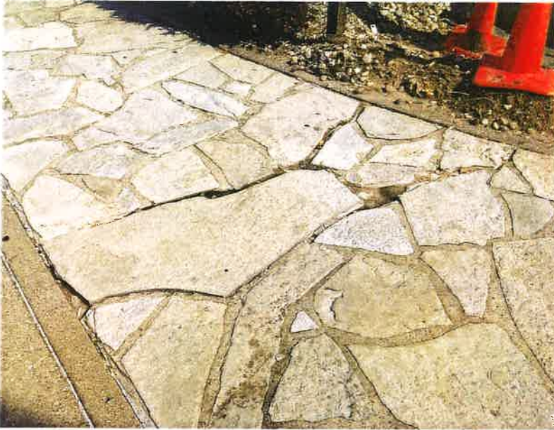
Missing mortar / loose stones
