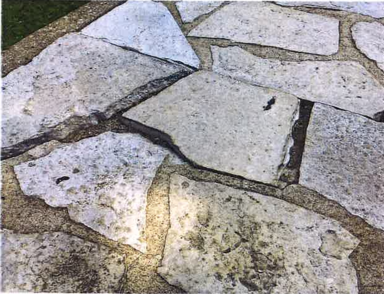
Missing mortar / loose stones
