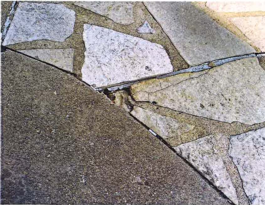
Missing stone and mortar
